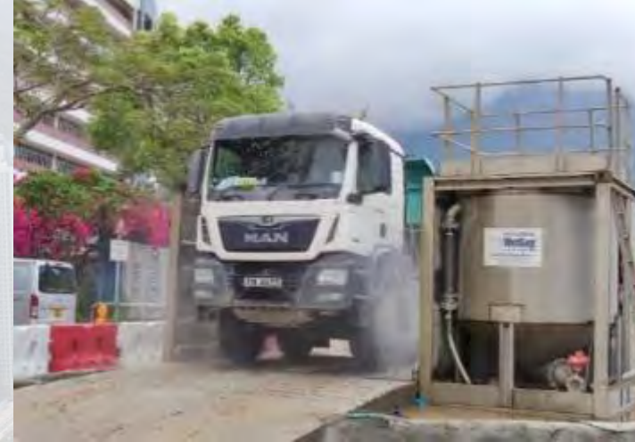
Wheel washing facility at the site exit
